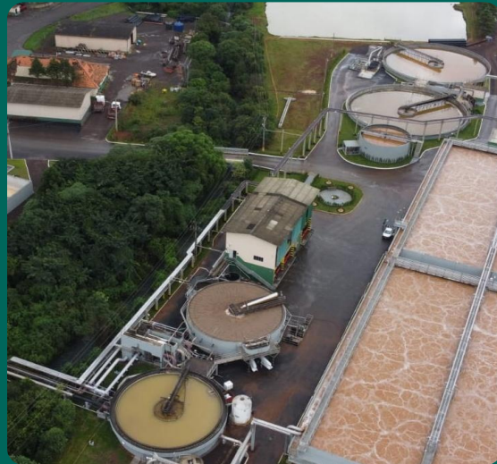
EFFLUENT TREATMENT PLANT CDM
