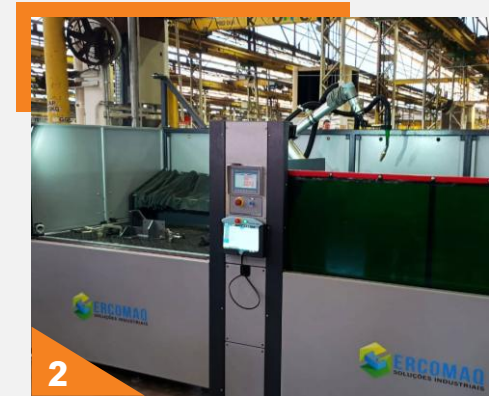
(2) Collaborative Welding Cell (Collaborative Robots).
