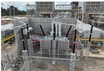
UTE: Backfeed GTG 11
