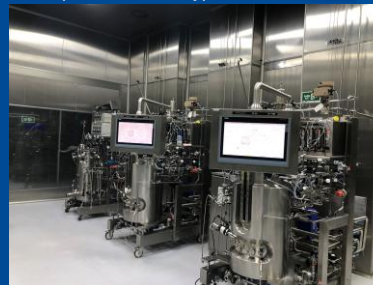
P400 (Blau API Facility)
