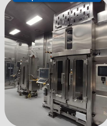
3,000 liter reactor for the production of mAbs
