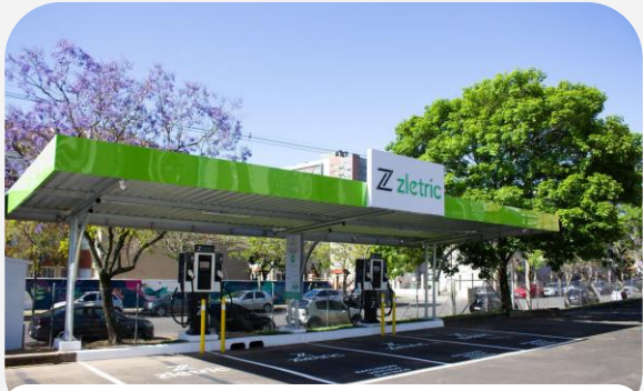
PORTO ALEGRE – RS Charging Station Parque Germânia
